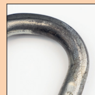
Superficial corrosion to the steel
